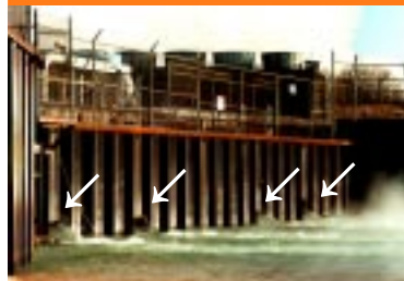
Water discharge area at Palisades Nuclear Power Plant on Lake Michigan. Note the flow from four big ejection outlets.
