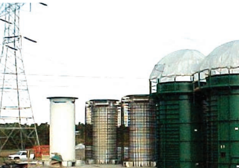
Image of dry spent fuel casks on concrete pad at a nuclear power plant site. (Nov. 2007)
